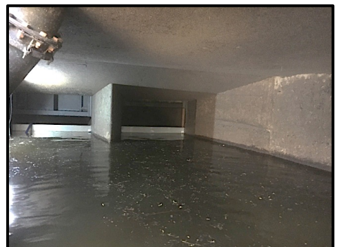
The bottom right photograph is looking towards the turbine inlets where aluminium plates have been installed to hold back water.
